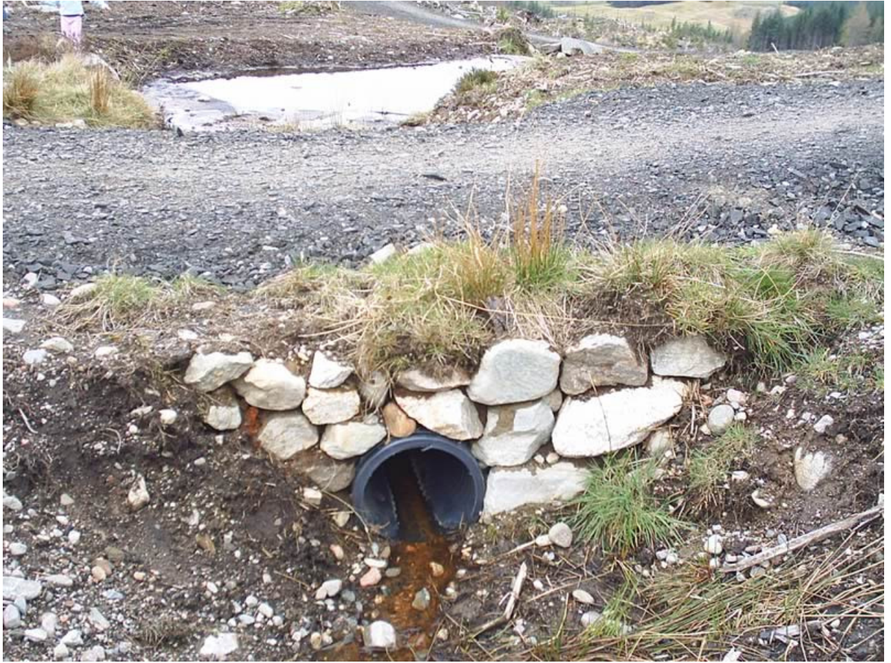
A typical example of a piped culvert with a headwall built using dry bonded stone and turfed to blend in.
