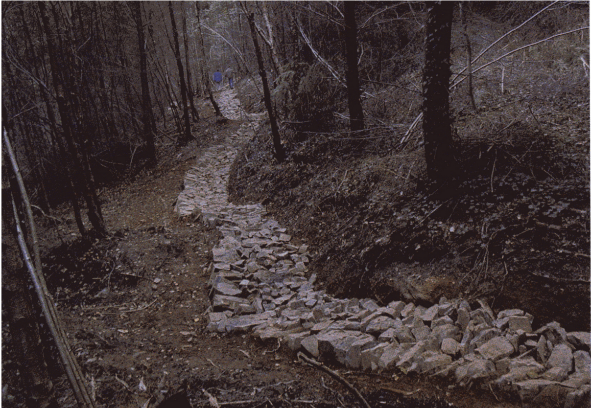
A typical stone fill example prior to the surface coat being applied i.e. the finer material.
